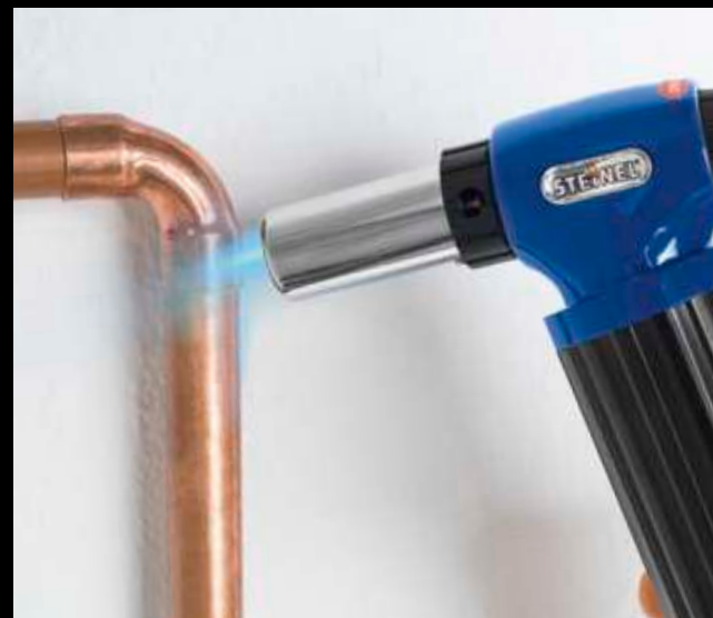
Solder joints on copper piping
